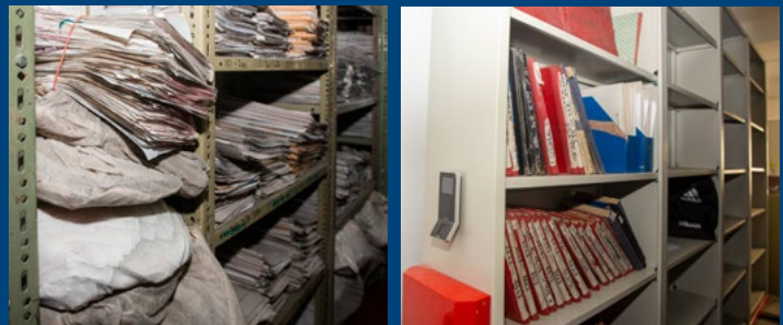
File storage before and after repositories installation. Photo credit: MTaPS Nepal
